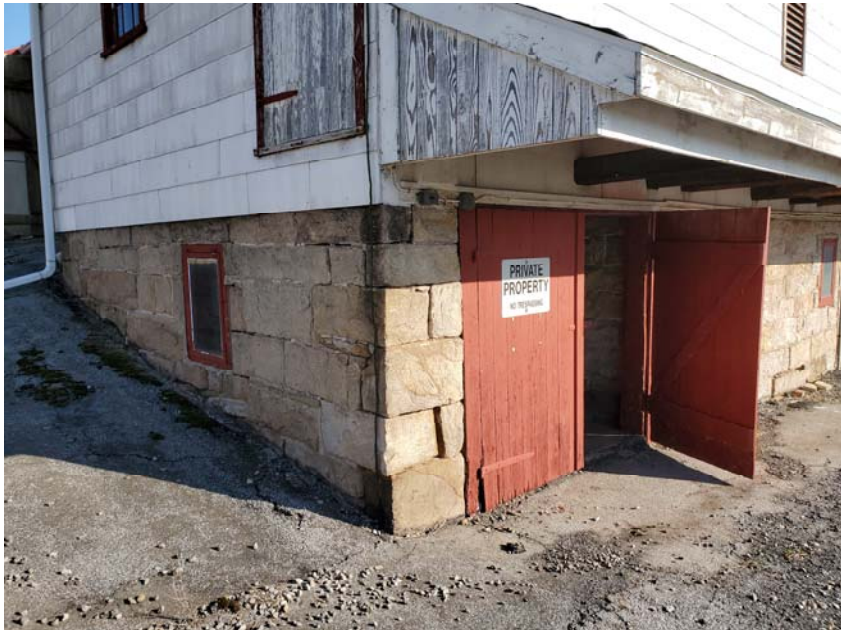
Stone in Need of Repair at North-East Corner
