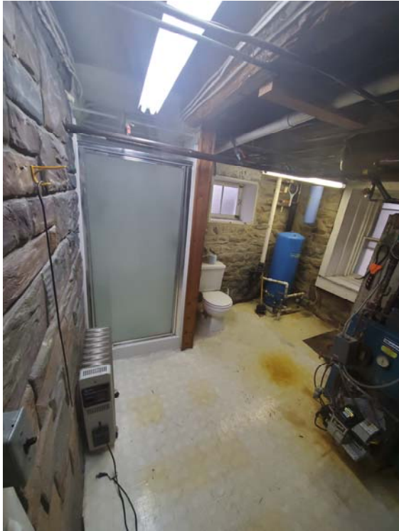
Basement Level - Utility Room
