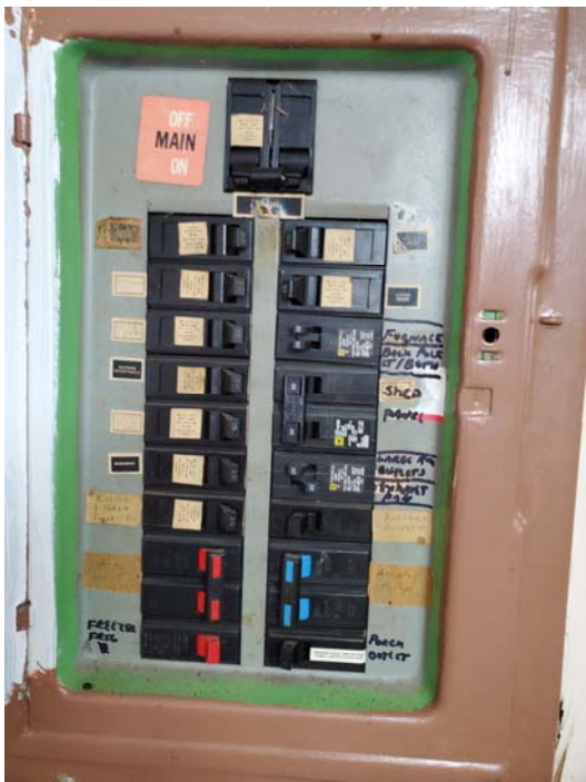
Detail of Electrical Panel
